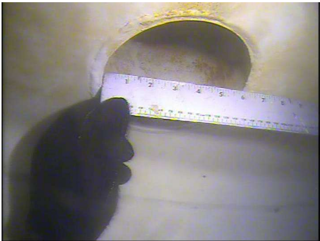
Common Inlet/Outlet – Staining Noted
