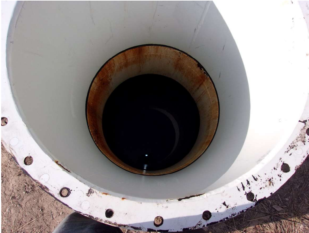
Access Hatch – Coating Failure with Corrosion Noted
