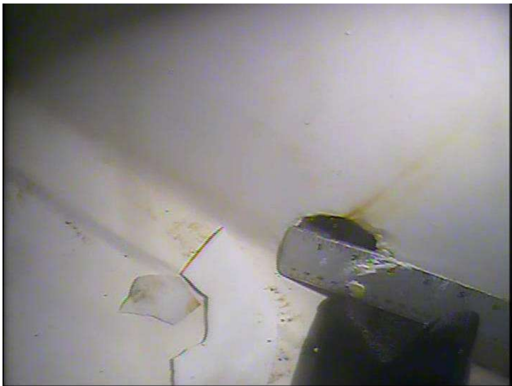
Drain Plumbing – Coating Failure with Corrosion Noted
