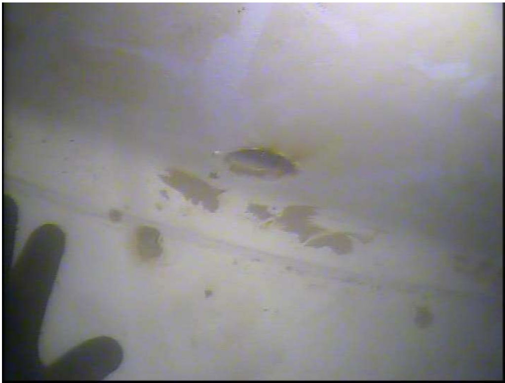
Common Drain – Coating Failure with Corrosion
