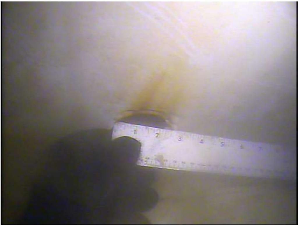
Drain Plumbing – Coating Failure with Corrosion Noted
