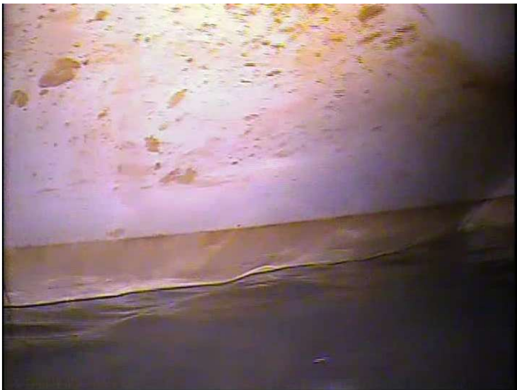
Wall to Roof Seam – Staining Noted
