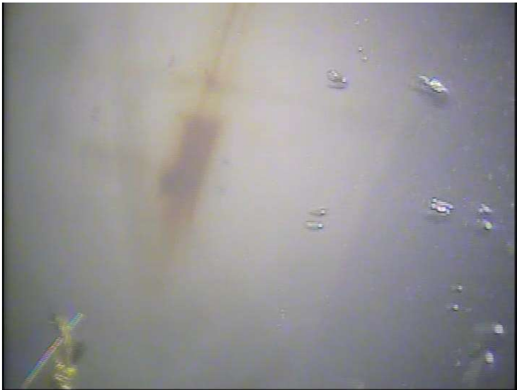
Typical Wall – Coating Failure with Corrosion
