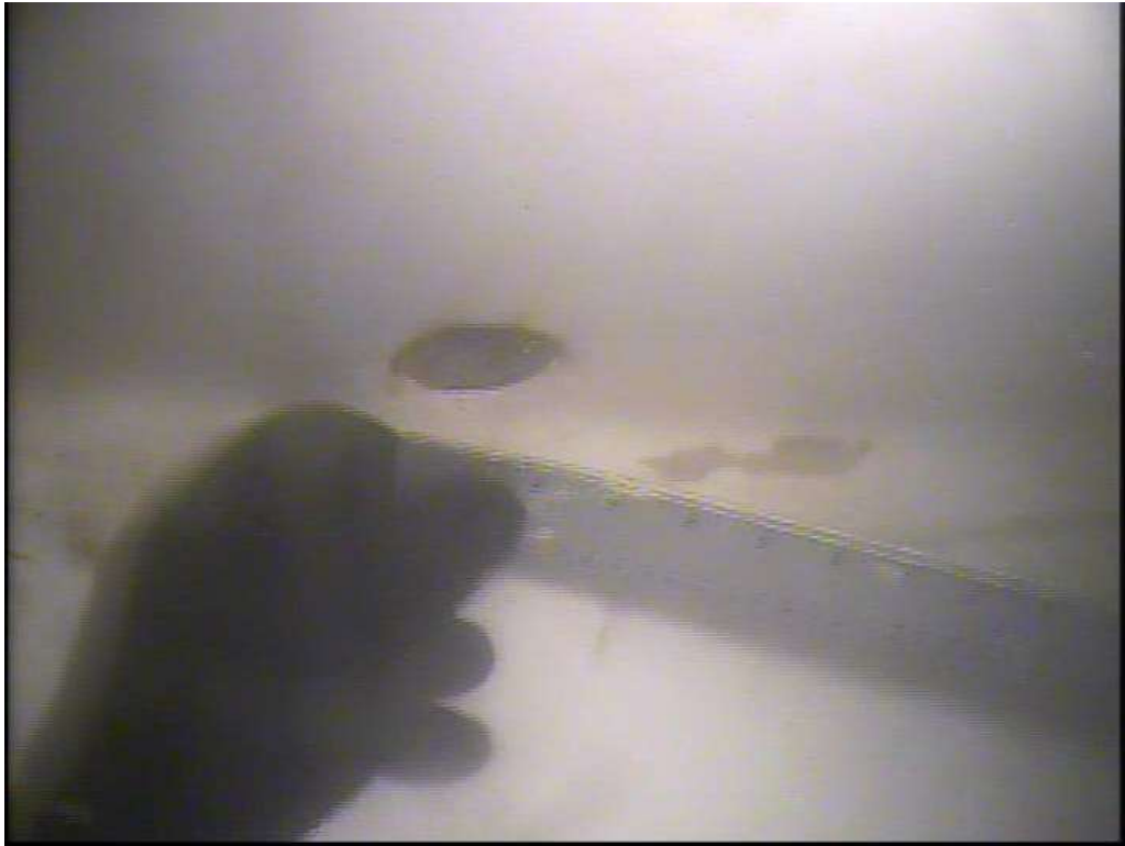
Drain Plumbing – Coating Failure with Corrosion Noted
