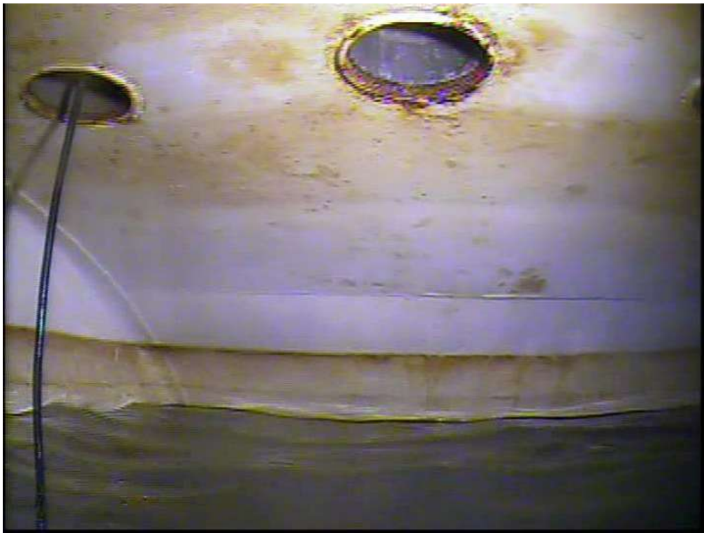
Interior Plumbing – Coating Failure with Corrosion
