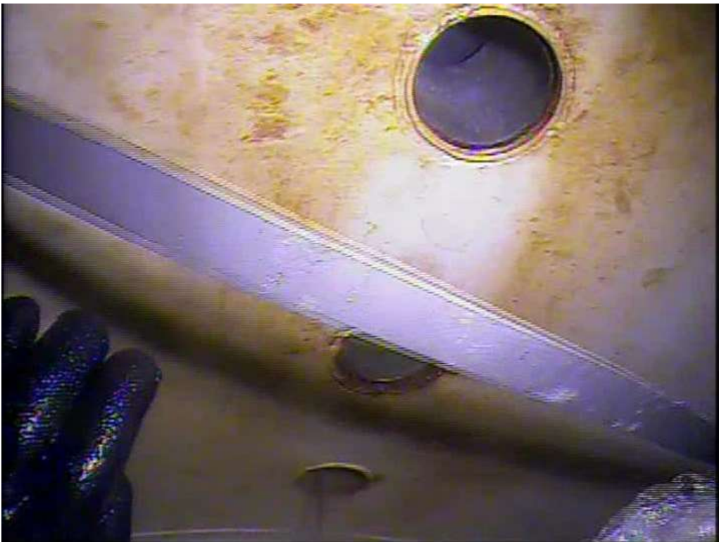
Overflow Plumbing – Coating Failure with Corrosion Noted
