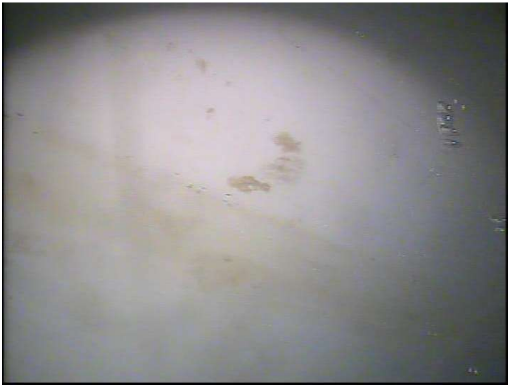
Typical Wall - Staining Noted
