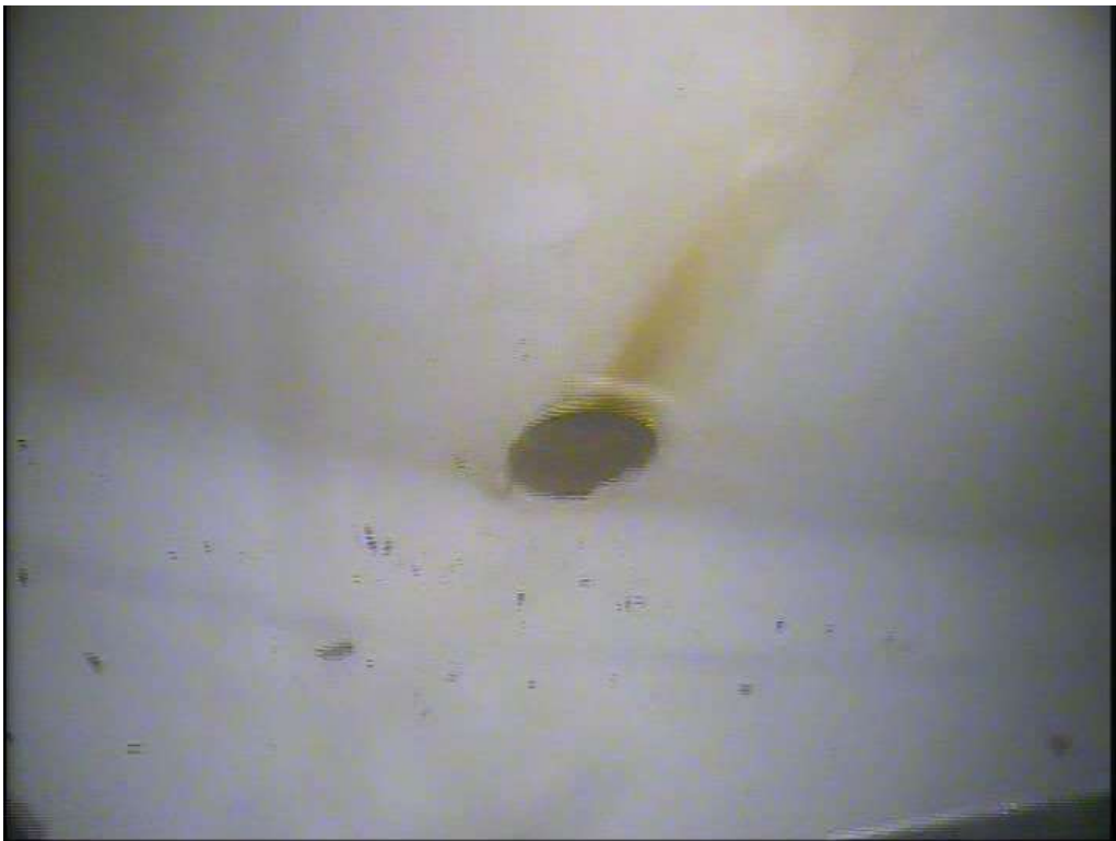
Drain Plumbing – Coating Failure with Corrosion Noted
