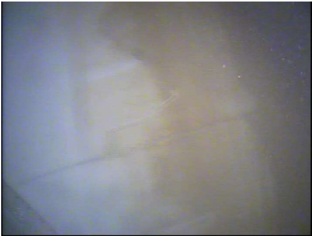
Typical Wall – Staining Noted
