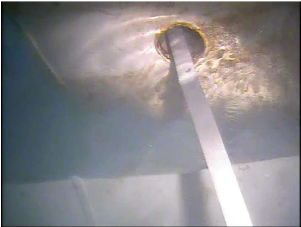
Overflow Plumbing/Roof Vent – Staining Noted
