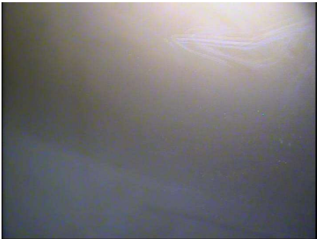
Floor to Wall Seam
