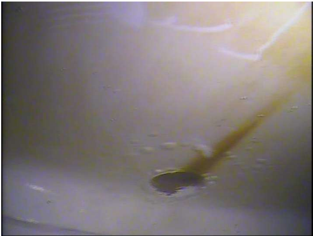
Drain Plumbing – Coating Failure with Corrosion
