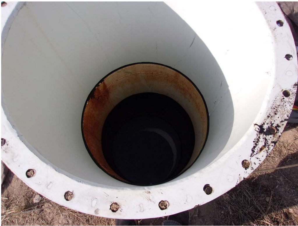
Access Hatch – Coating Failure with Corrosion Noted
