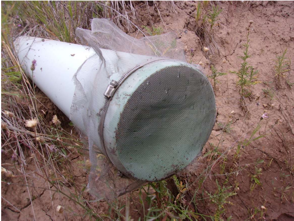
Overflow Plumbing – Screen Deterioration Noted
