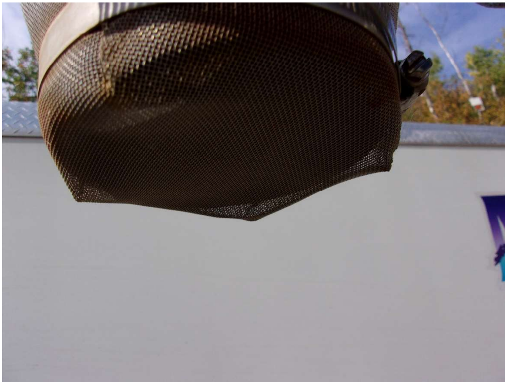
Roof Vent Screen - Staining Noted
