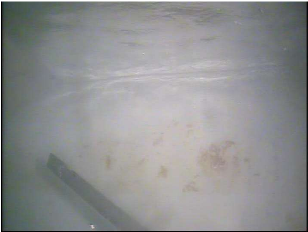
Typical Wall – Staining Noted
