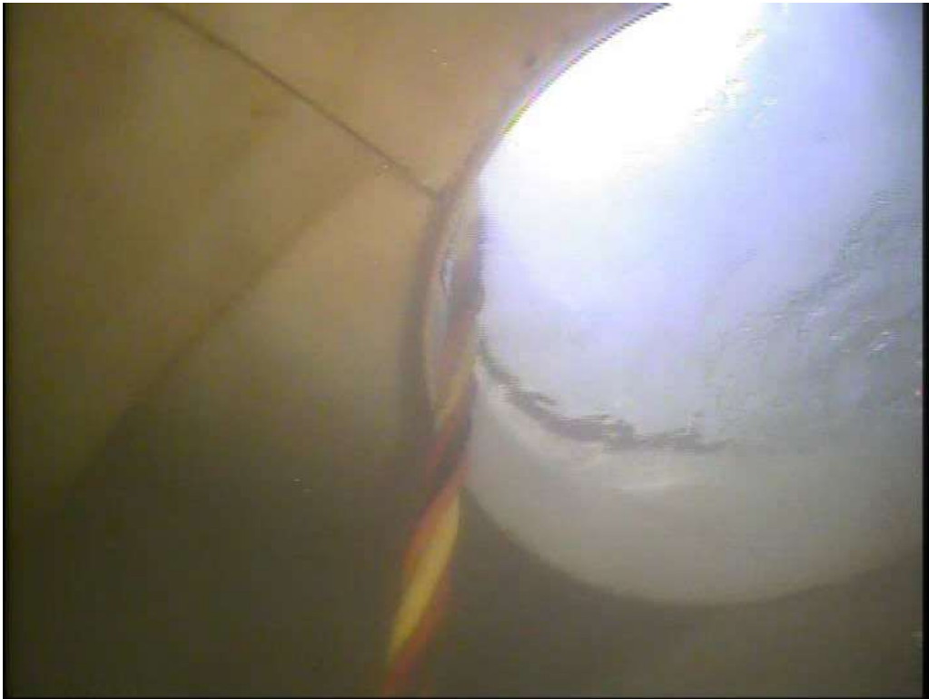
Access Hatch – Staining Noted
